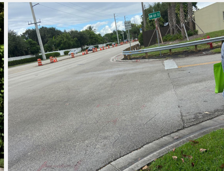
Guardrail installed keep speeding vehicles from crashing into properties at NW 68th St
