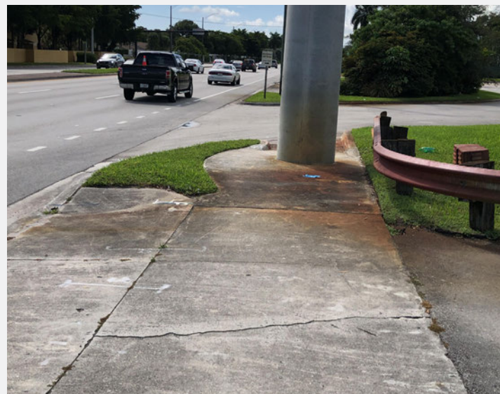
Power pole obstructing sidewalk south of Middle River
