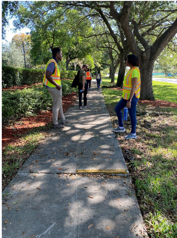
Uneven sidewalk on eastside of corridor.
