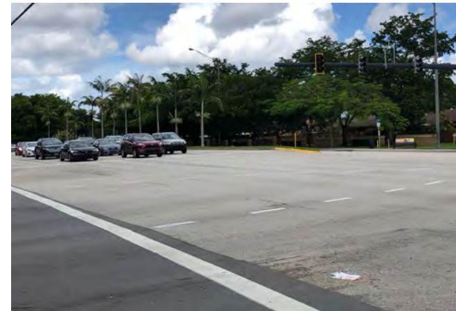
University Dr: The eastern end of Cleary Blvd. Crosswalk missing over University Dr.
