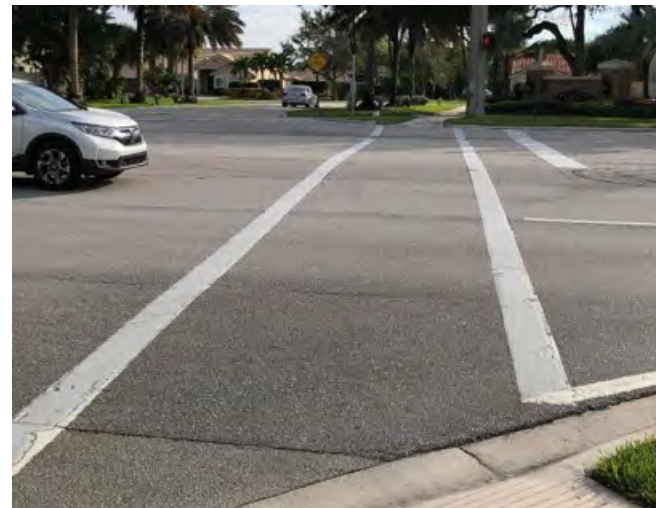
NW 12th St intersection (NW view); Typical infrastructure and no left turn signal on cross-streets.
