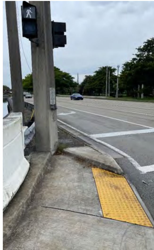
Broward Bl intersection. SW corner curb is very narrow due to canal.
