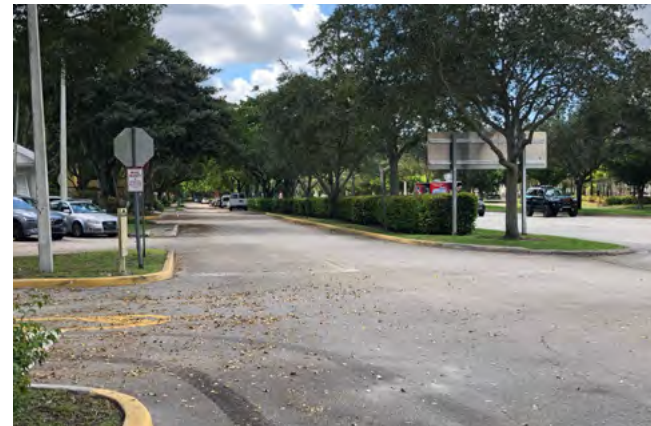
NW 79 Te: University Dr's sidewalks are located here. There are sidewalk gaps, no crosswalks, and non-ADA compliant curbs.
