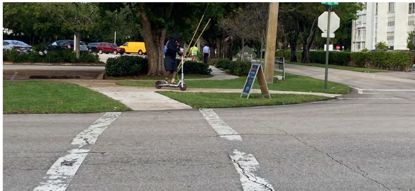
SE corner of Cypress Rd and NW 69th Av (west view); Faded crosswalks and adjacent sidewalk veers into parking lot.
