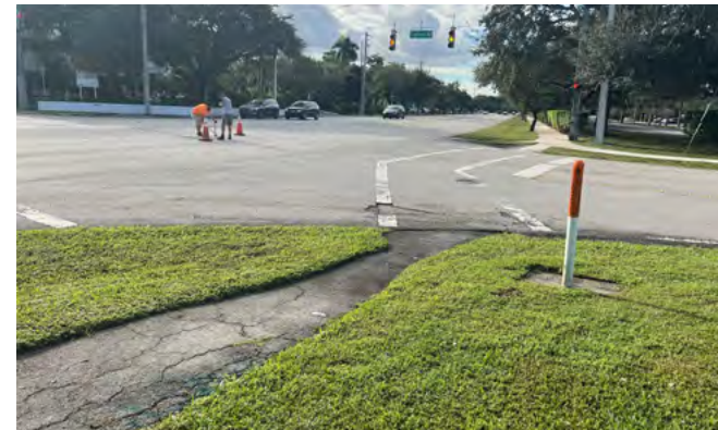
Cypress Rd and NW 70th Av intersection (west view); Cypress Rd widens to include striped median. Curbs and crosswalks are in poor condition.
