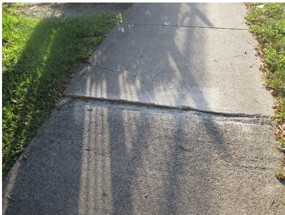
Cracked sidewalk/trip hazards along the sidewalks.
