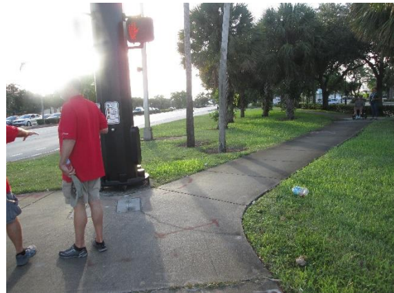
Some locations of the pedestrian signal push buttons are not ADA compliant due to the distance from curb ramp.
