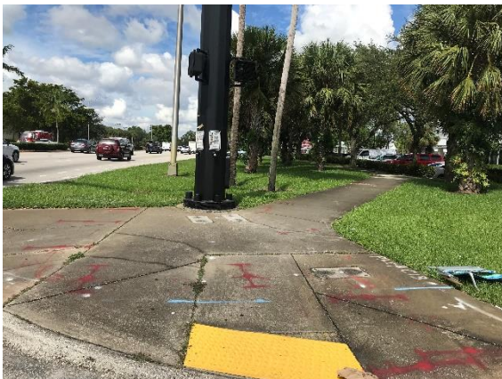
Evaluate the push button location to make sure it is following minimum ADA requirements and evaluate the ADA detectable warnings.
