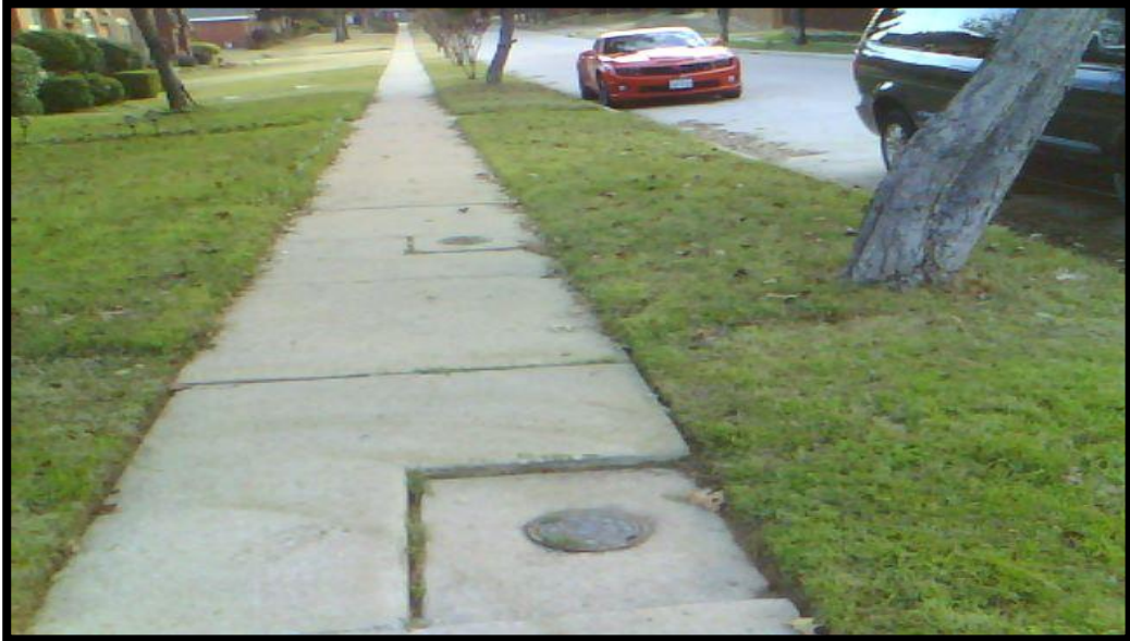
Sinking, utility obstruction
