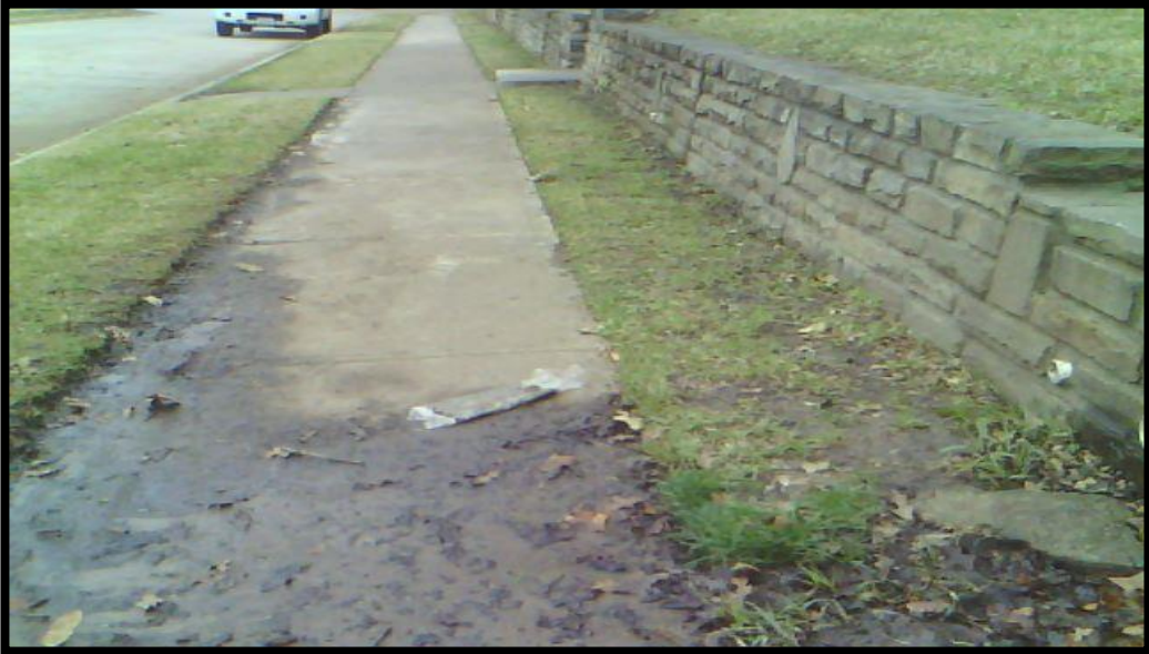
Ponding, temporary obstruction
