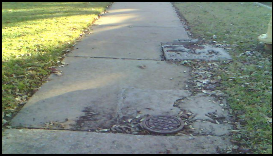
Cracking, utility obstruction
