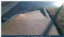
MISSING DETECTABLE WARNING SURFACE
