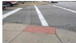
POOR ALIGNMENT WITH CROSSWALK
