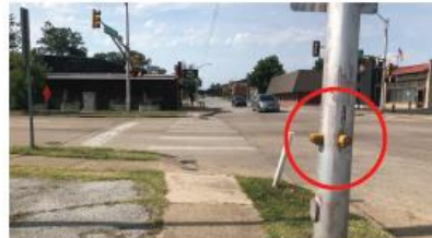
MISSING PEDESTRIAN CROSSING SIGN
