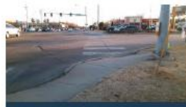
NO LANDING AT TOP OF CURB RAMP
