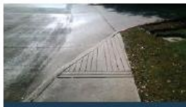
STEEP CURB RAMP CROSS-SLOPE
