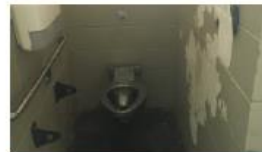
NON-COMPLIANT PARK AMENITIES
