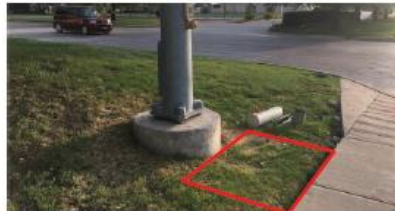
NO ACCESS TO PUSH BUTTON
