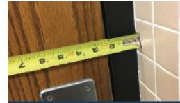
NO DOOR MANUEVERING CLEARANCE
