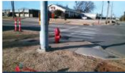
OBSTRUCTION IN CURB RAMP
